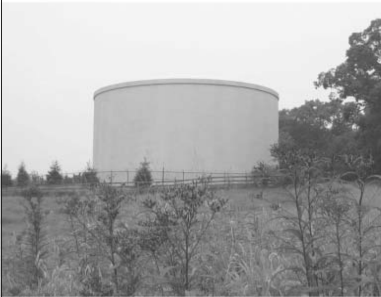
2.0 MG water storage tank in Sellersburg, IN for the Silver Creek Water Corp. Engineering by Jacobi, Toombs & Lanz, Inc.
